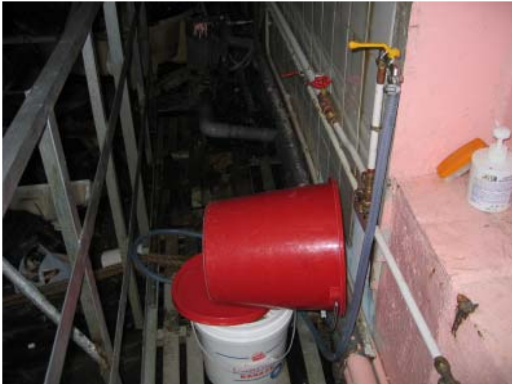
Picture 4. Temporary water supply outside the window of the elderly home in the morning of 4 September
